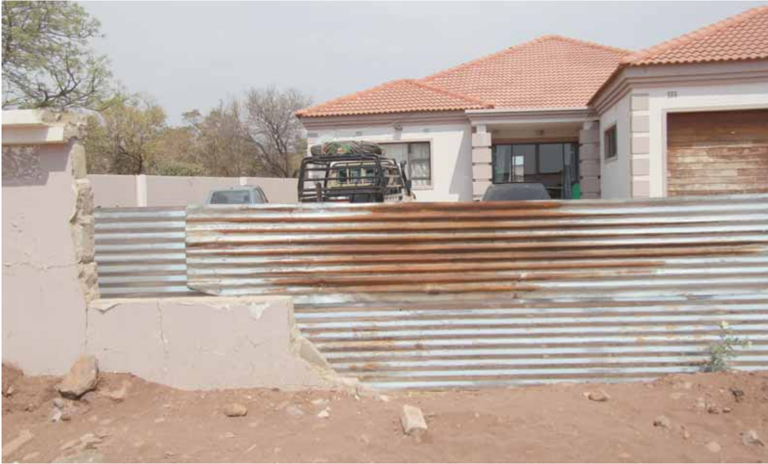
One of the homesteads damaged during the construction of Kanye Sanitation Project. Minister of Water, Sanitation and Human Settlement, Mr Onneetse Ramogapi told the Kanye District Full Council meeting on Tuesday that costs escalation incurred by government on the project from P700 million to P3 billion was justifiable. Photo: Thandy Tebogo
