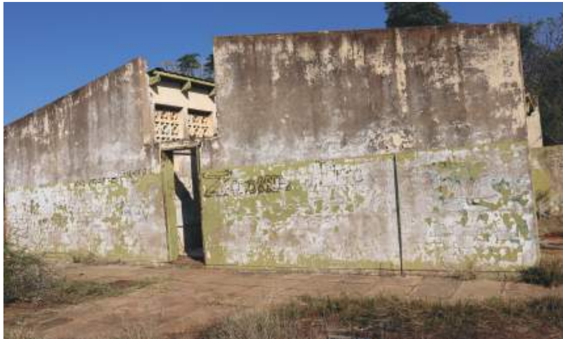
Molefhi Senior Secondary School old toilet block that has turned into crime haven where learners hide to smoke. Photos: Mmoniemang Motsamai
