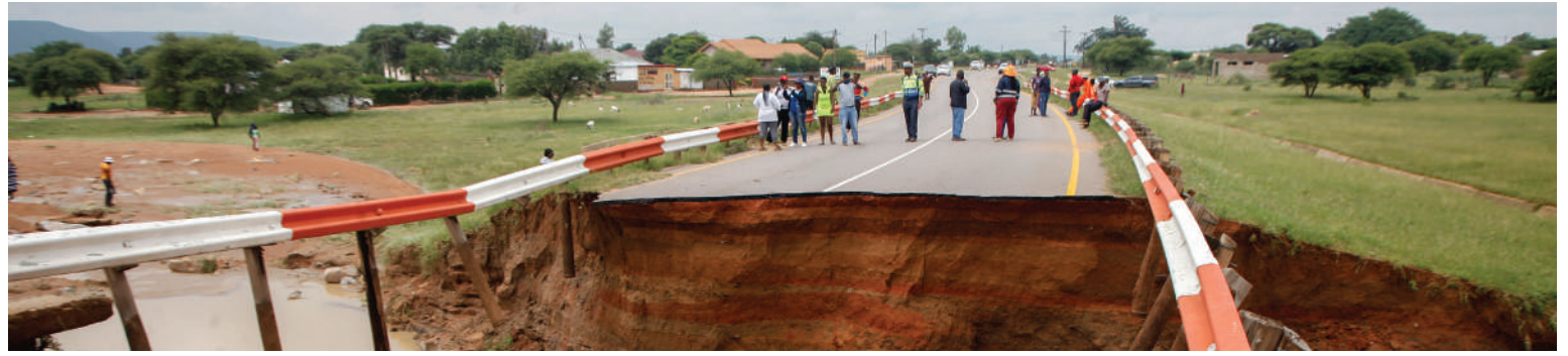
Moshupa A10 bridge, which has been closed due to severe structural failures and complicated underground water conditions, has been thrown a P12 million lifeline. Senior district officer for development, Mr Tebogo Mekwe said a contract had been awarded to Herbco Technical Services (Pty) Ltd for detailed investigation, as well as pre- and post-contract engineering services, to permanently resolve the bridge's ongoing structural issues.
