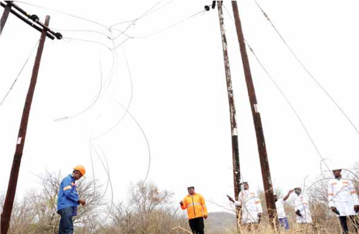
Botswana Power Corporation is reportedly overwhelmed by a problem of electric power cable theft and vandalism of infrastructure, which are exacerbated by a readily available black market. The corporation has recorded over 100 households that have been affected by power cable theft in Maun.
