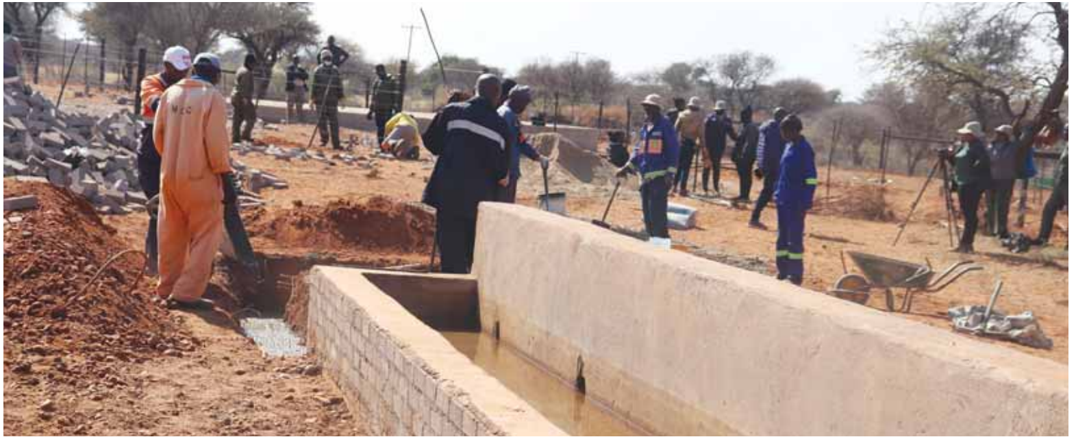
Loporung residents constructing a water reservoir and drinking trough for livestock. The project is part of the 14 projects to be undertaken in villages along the Molopo River following government's decision to construct a cordon fence from Tlhareselele to Mabule.
