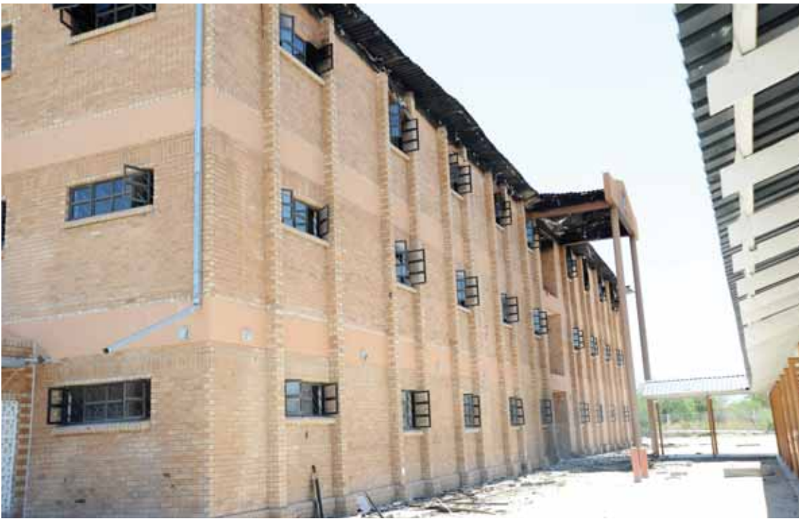
Minister of Child Welfare and Basic Education, Ms Nono Kgafela-Mokoka said the ministry would spend P145 million on major restoration works at Nata Senior Secondary School in the second quarter of the 2026/27 financial year to address fire damages and the facility's aging infrastructure.
