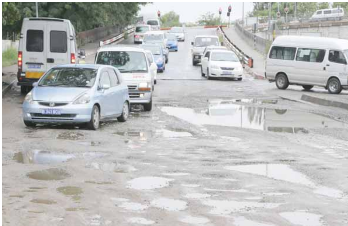
The City of Francistown Council uses over P1 million on average to maintain internal roads.
