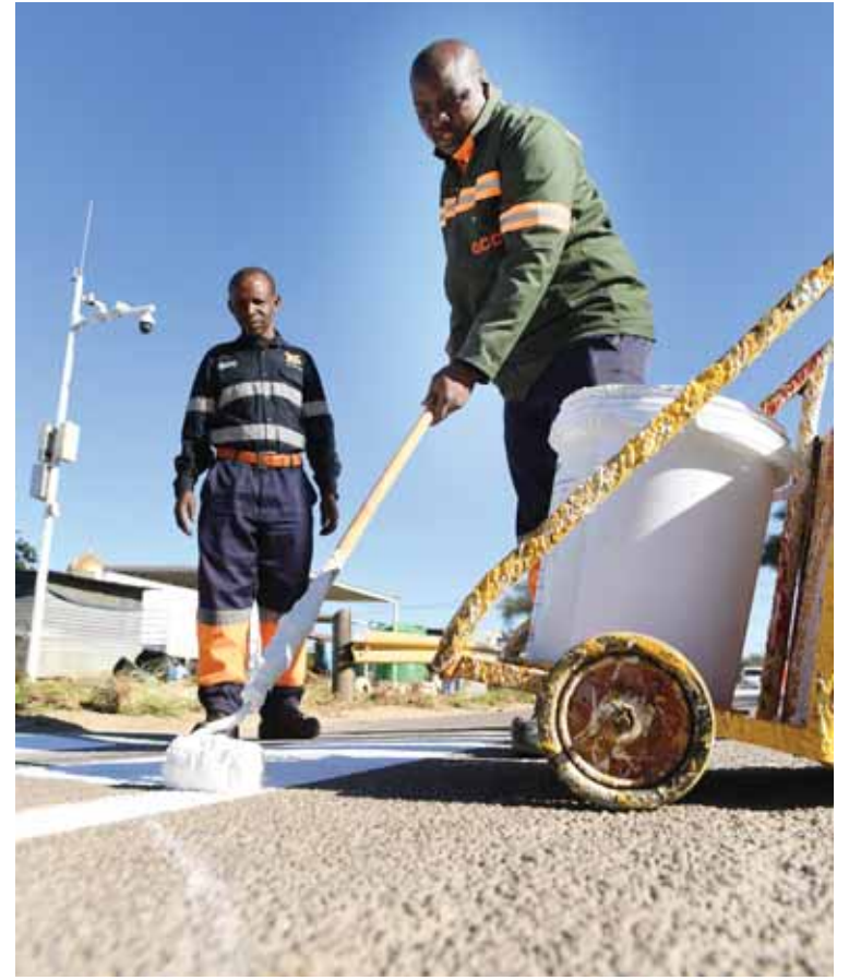
Gaborone City Council employees painting road markings at Tshweneng Ward in Gaborone on Saturday. The council has embarked on a City Upkeep exercise to enhance the general environment and ultimately promote sustainable urban cleanliness.
