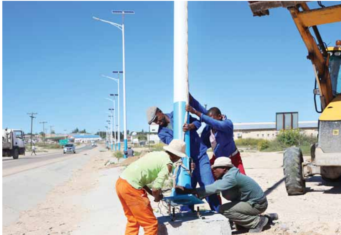
Electricians installing street lights. Addressing Moshupa District Council, Mr Phiri pleaded with communities to guard against the new type of crime in which infrastructure, especially the solar street lights were being knocked down by motorists so to steal them for domestic use.
