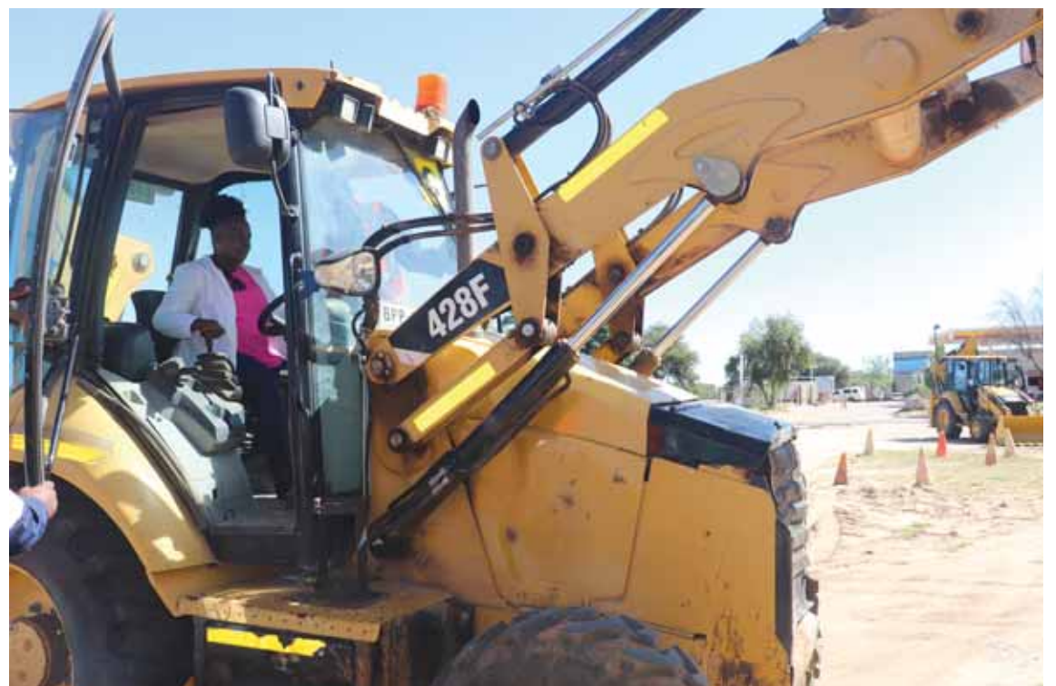
Jwaneng mayor, Ms Olga Ditsie performing the official ground-breaking for the town council's road maintenance projects worth over P6 million. Photo: Kehumile Moekejo
