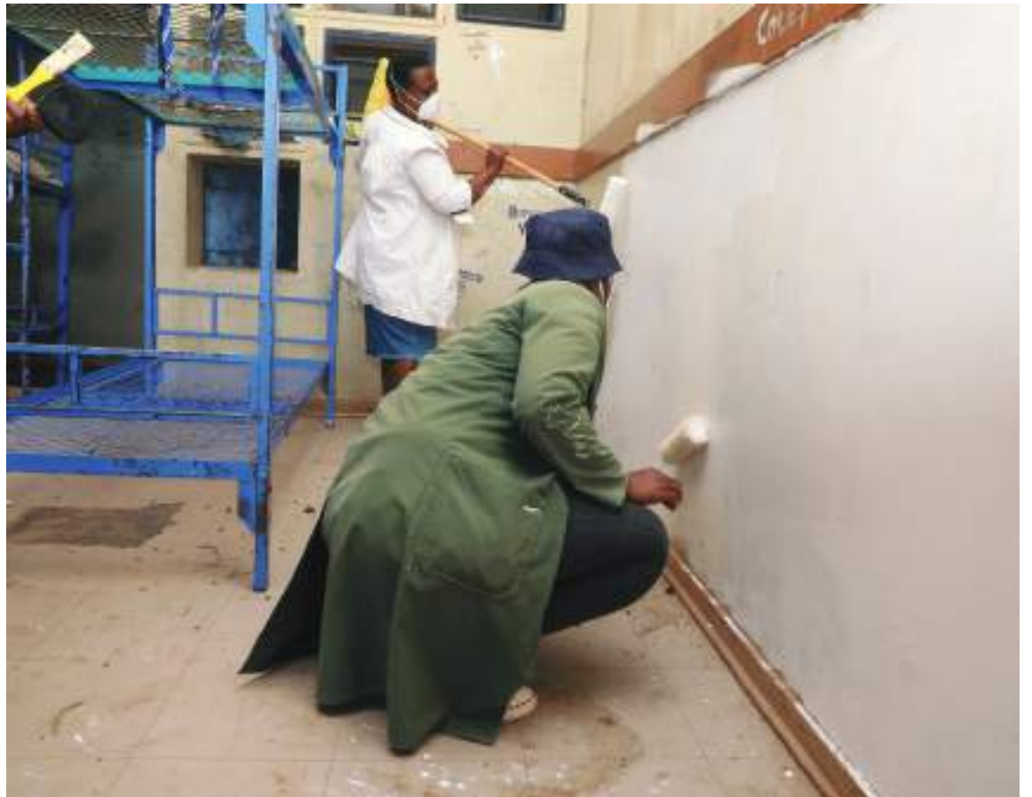
Mabeleapudi residents participating in the renovation of hostels at Patikwane Junior Secondary School on Saturday. The project was spearheaded by Serowe North Member of Parliament and Assistant Minister of Trade and Entrepreneurship, Mr Baratiwa Mathoothe, under the: Motho le Motho Setena initiative. Photos: Baldwin Nyamande
