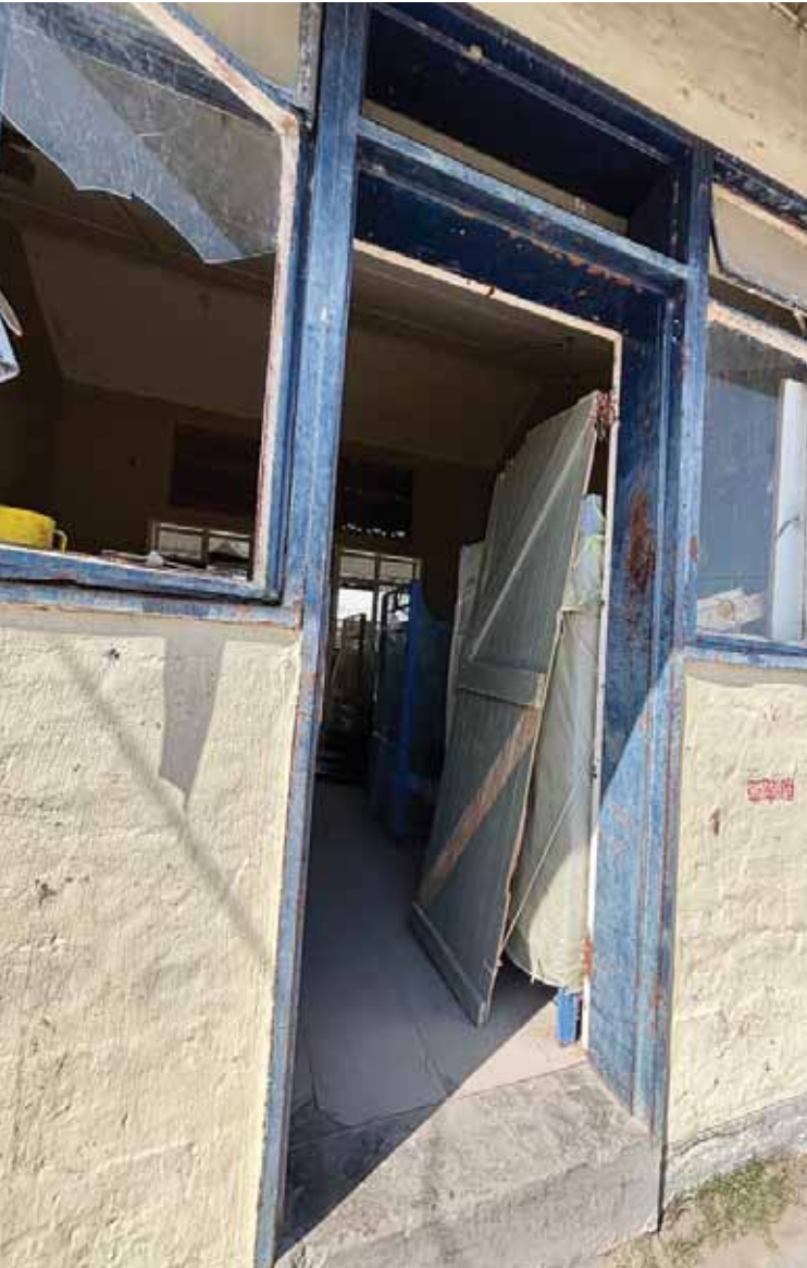
Hostels, classrooms and ablution facilities were in poor condition.
